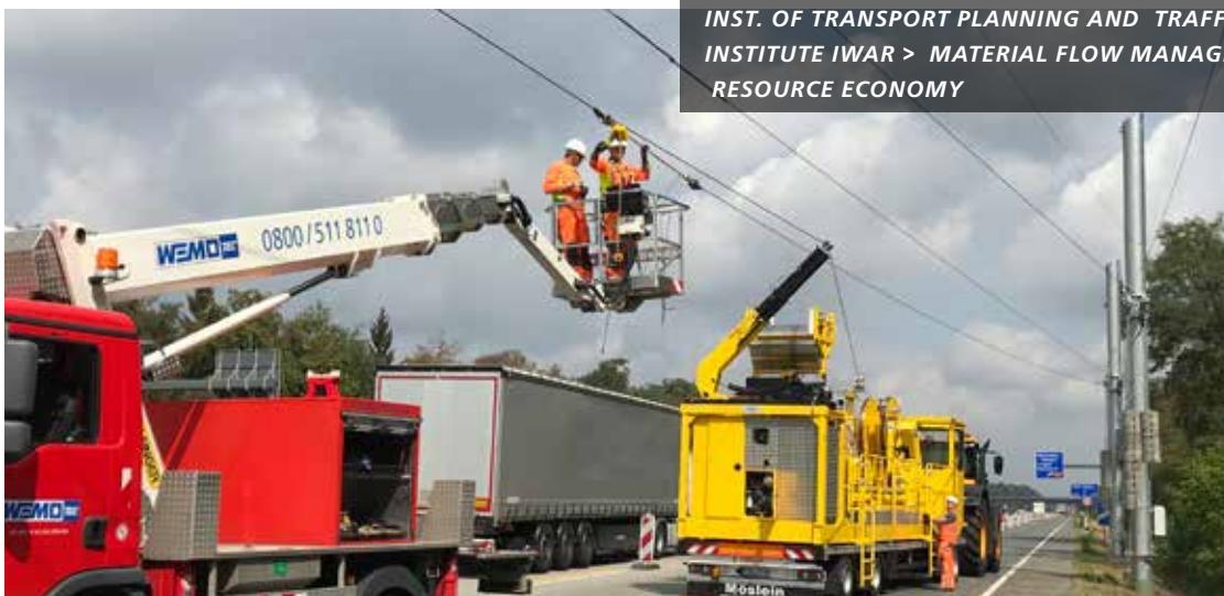
BAUARBEITEN AN DER A5 construction work on highway A5 (source and copyright: Hessen Mobil)
